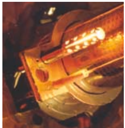
Hot surface ignitor and flame probe.
